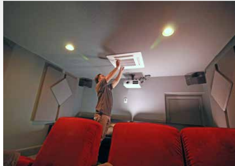
To give precise and responsive control over the basement theater room, Sharp installed a ceiling cassette unit with its own thermostat.
