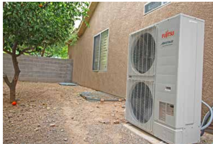
The 4,000 square-foot home needed a five-ton VRF system to replace the air conditioner and gas-fired furnace.
