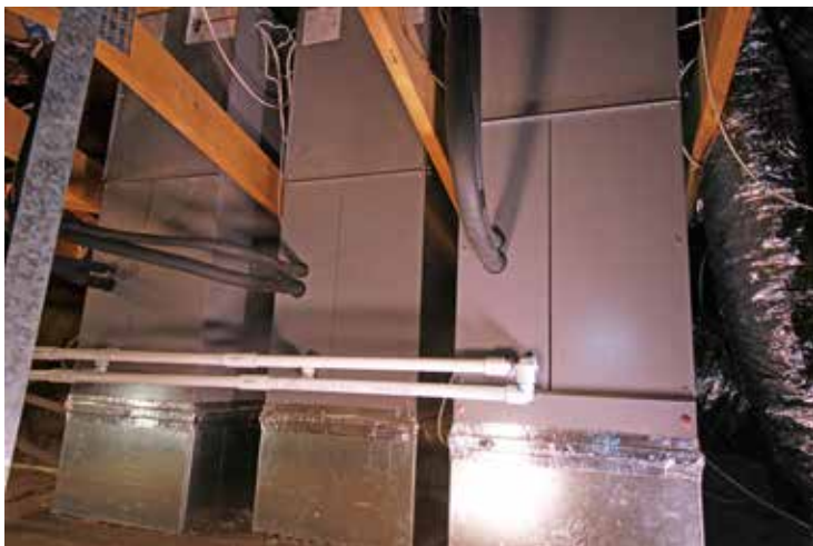
The large trunk line and coil in the attic was removed and replaced by three smaller branches and fan coils supported by the VRF condenser outside.
