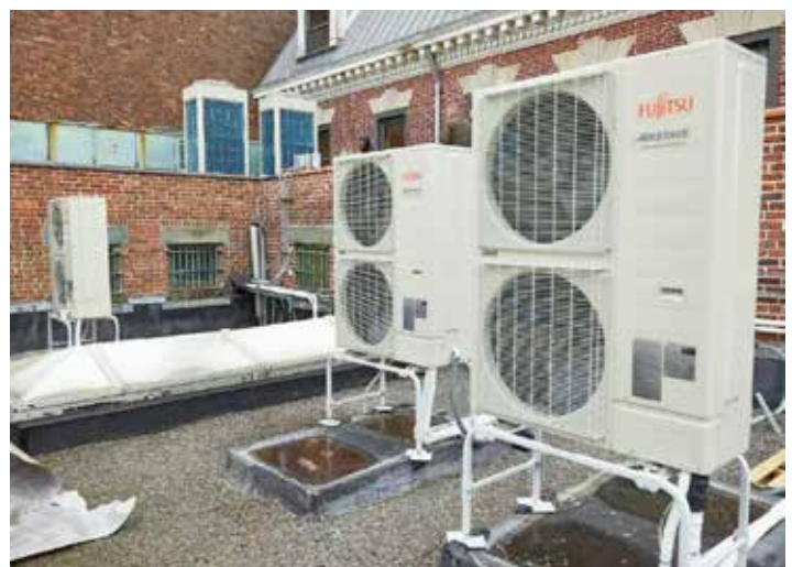
A variety of Airstage VRF and Halcyon mini-splits were used by DCAS to replace a steam heating system
