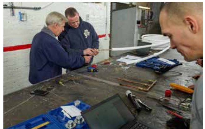
All facets of VRF installation are taught to DCAS employees at the Henry Chang Learning Center.
