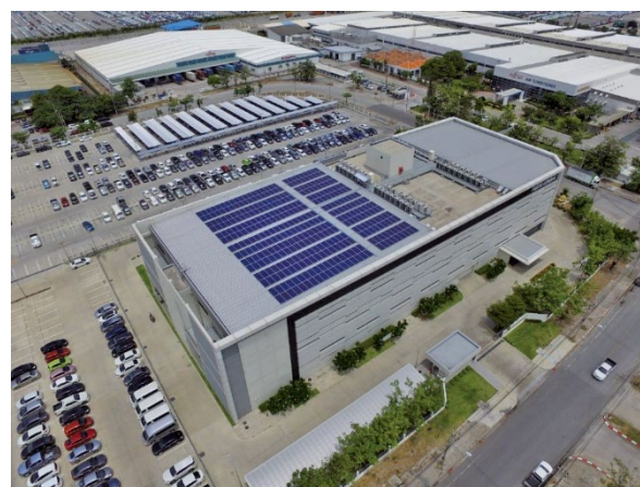
R&D center in Thailand Solar panels installed for self-consumption
