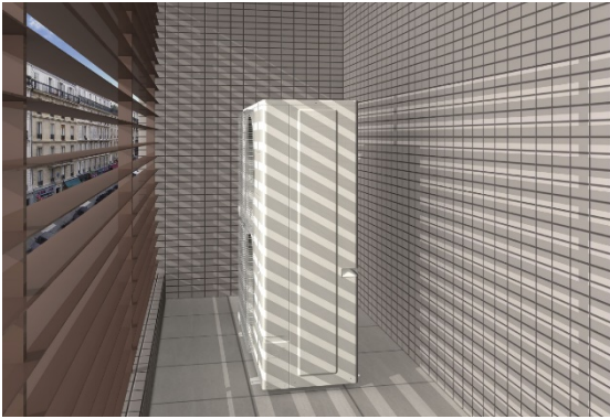
J-III L (18HP) installed on a balcony covered by an external louver (Image)
