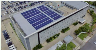
Solar panels were installed on the roof of our R&D Center in Thailand
