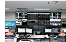
Fire and emergency communication command system
